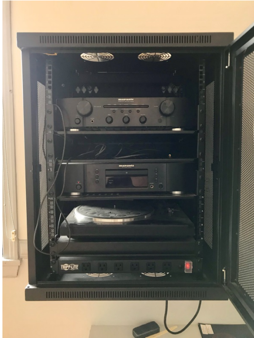
Audio cabinet at front of house right
